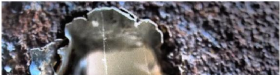
Peeling paint from Eastern State Penitentiary hospital wing (also framed shot)
